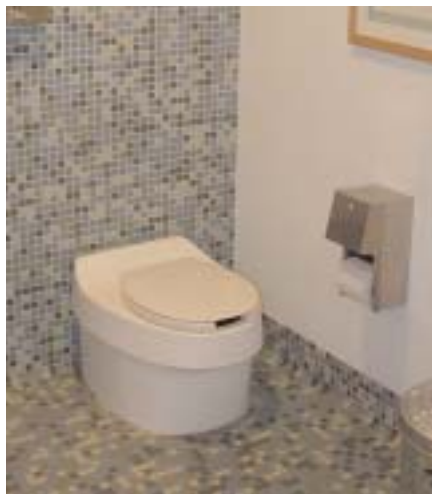
Composting toilets save water at the Chesapeake Bay Foundation's Philip Merrill Environmental Center.
