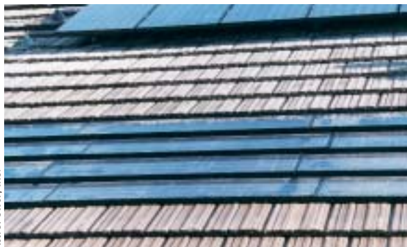
AstroPower's new solar array aligns with existing roof shingles.
