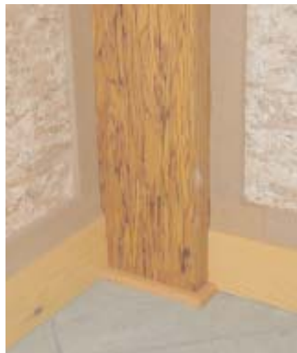
The exterior timber framework of the Philip Merrill Environmental Center is constructed of parallel-strand lumber, which is made from small-diameter trees.
