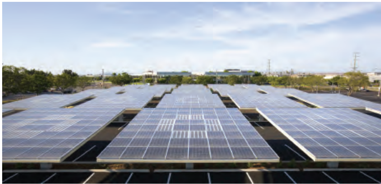
Kyocera's 235-kilowatt solar carport, or Solar Grove, is located in San Diego at Kyocera's North American headquarters.
