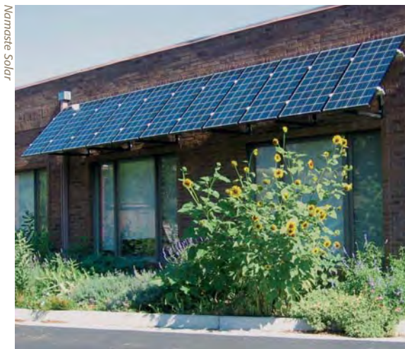
The PV awning system Namaste Solar Electric donated to KGNU Community Radio helps offset the station's operating expenses.
