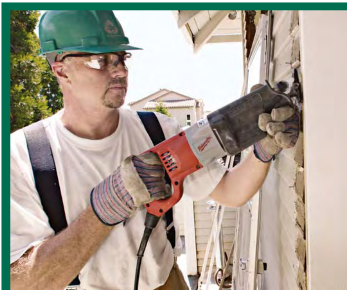
A reciprocating saw is an essential tool on a deconstruction site for cutting nails and wood, especially in tight places.
