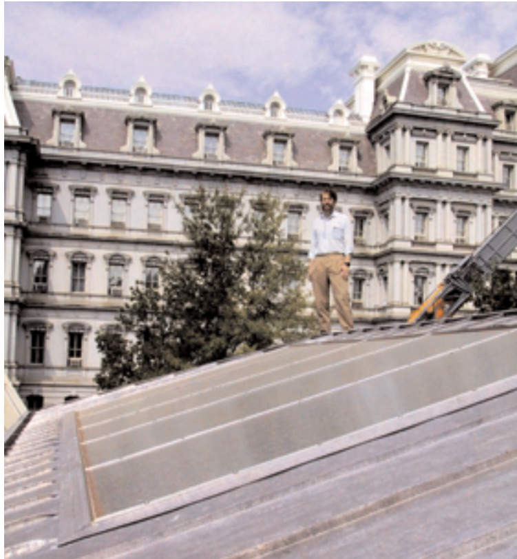
The solar thermal array is integrated into the historically correct, lead-coated copper, standing-seam roof on the White House pool cabana. The site-fabricated assembly uses selective-surfaced absorbers from SunEarth.
