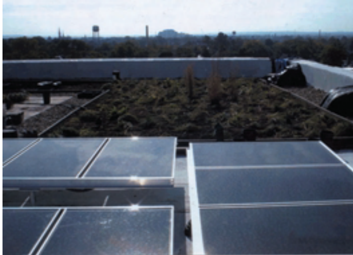
StressPly® EUV was recently installed on the roof of the Cleveland Environmental Center in Cleveland, Ohio, along with Garland's GreenShield™ green roof, SolarGrid™ photovoltaic rooftop panels and White Knight™ urethane coating.
