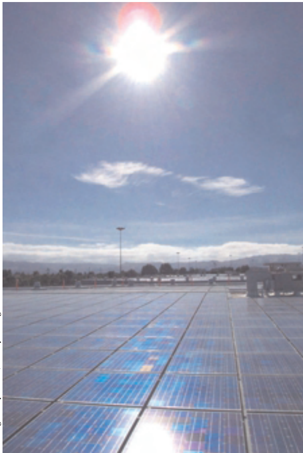
The 1.18-MW PowerLight PV system on the roof of the Santa Rita Jail in Dublin, California, covers about 3 acres of the jail's roof.
