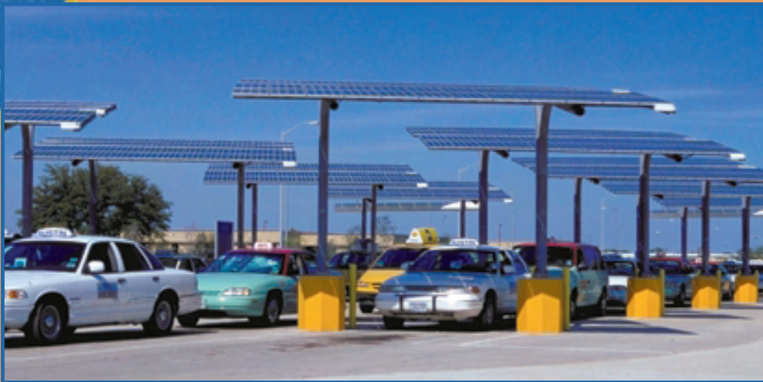
Austin-Bergstrom International Airport Taxi Stand Project, 26.4 kW (2000)
