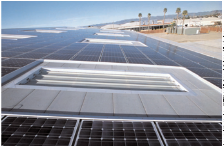
A series of skylights mounted between the photovoltaic modules on the east-facing roof provide daylight to the production area of the Hayward plant.
