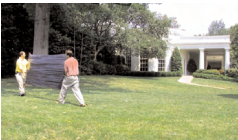
Solar installers carry an absorber plate by the oval office to be installed on the first family's pool cabana adjacent to the west wing.
