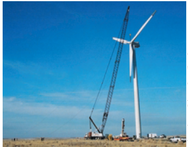
Crews install this 750-kilowatt NEG Micon wind turbine on the Rosebud Sioux Indian Reservation in South Dakota.
