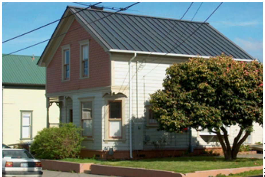
United Solar's building integrated photovoltaic standing seam roof replaces conventional roofing materials on this house in Historic Eureka, California.
