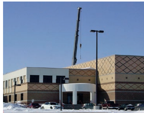
A crane stands ready to erect the wind turbine at Turtle Mountain Community College.
